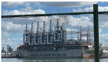
Karpowership says it currently has six 'Powerships' with an installed capacity of 420 MW in the country with a contract term for 18 years. Cuba is Karpowership's first project in Western Hemisphere. Crédito: Michael Adams
